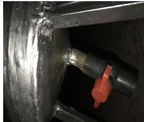
Figure 3: The outlet valve
