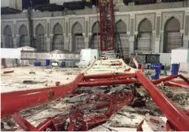
Fig. 2. the crane collapsed through the roof.
