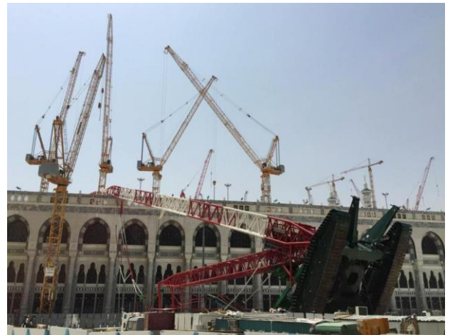
Fig. 1. deadly crane collapsed in Mecca, Saudi Arabia.
