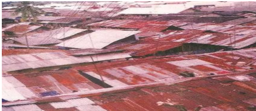
Figure 4: Corroded Building Roofs with Acid Rain.
