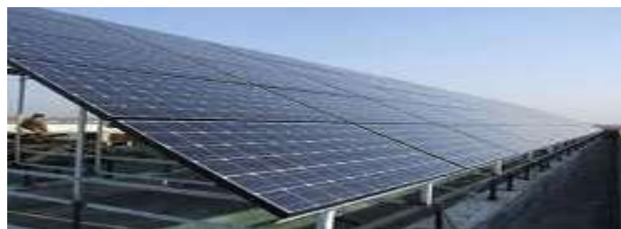
Figure: Solar photovoltaic system
