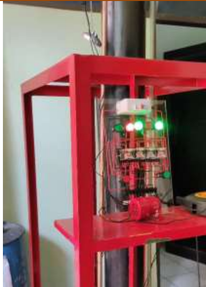
Figure 3. 2 System Test Filling Tank
