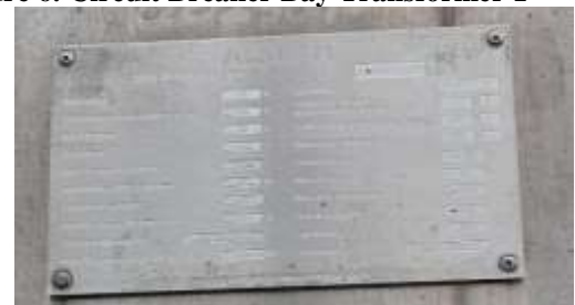
Figure 7. Transformer Bay Circuit Breaker Name Plate 1
