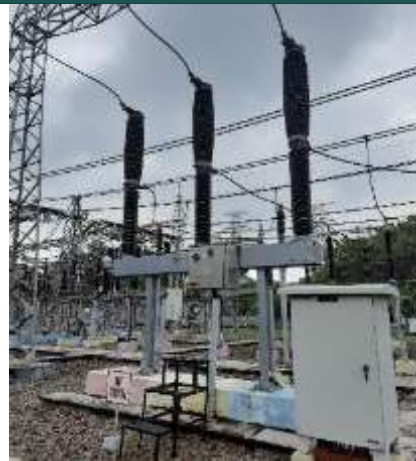
Figure 6. Circuit Breaker Bay Transformer 1
