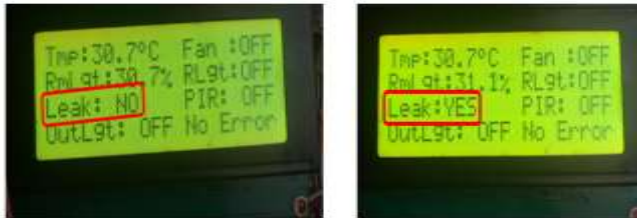
Figure 41 No gas leakage detected
