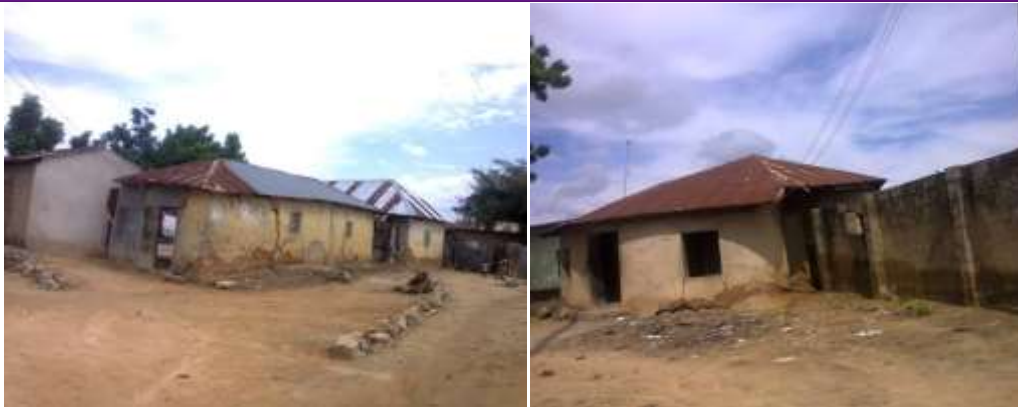
Plate I: The pictures show some of the walls constructed with mud block with signs of cracking.
