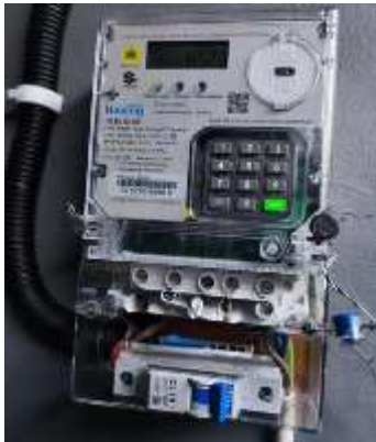
Figure 3: Typical electronic meter
